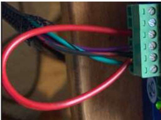
Figure 5 Color coding of the connections to the servo controller
